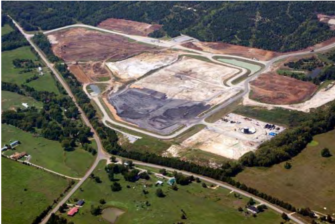
Figure 9: Arrowhead Landfill, AL, disposal of fly ash from TVA Kingston pond spill Photo courtesy of John Wathen, Hurricane Creekkeeper, Waterkeeper Alliance
