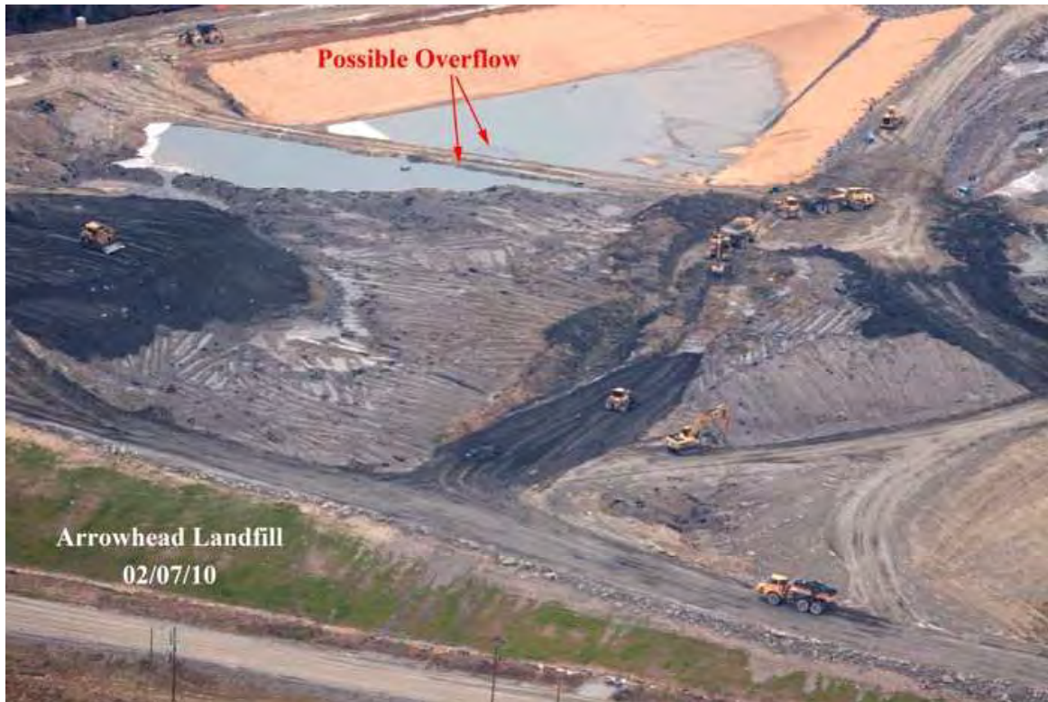
Figure 4: Fly ash management at Arrowhead Landfill, AL Photo courtesy of John Wathen, Hurricane Creekkeeper, Waterkeeper Alliance
