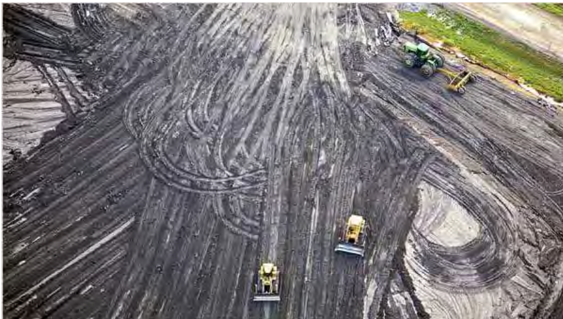
Figure 5: Fly ash management at Arrowhead Landfill, AL, From: New York Times, Clash in Alabama Over Tennessee Coal Ash, August 29, 2009; http://www.nytimes.com/2009/08/30/us/30ash.html?_r=2&ref=earth
